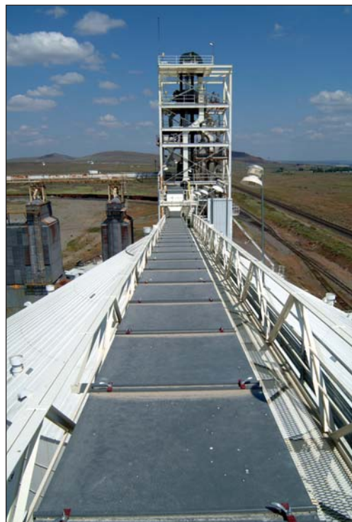
View along a new 40,000-bph Hi Roller enclosed belt conveyor back toward the head section of a new 40,000-bph Schlager receiving leg.
